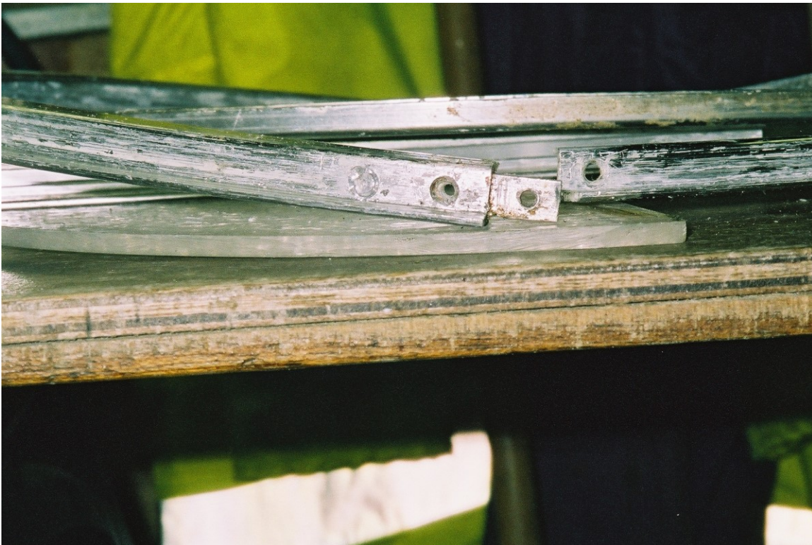
This picture shows where the frame comes apart and the old screws removed.
